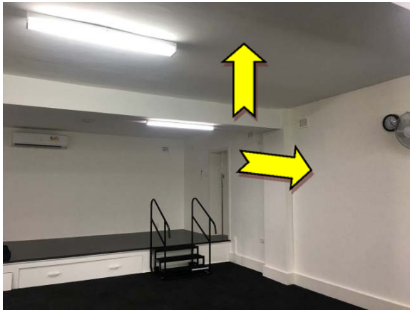
Photo 9. Interior, throughout, walls and ceiling – suspected lead-containing white upper paint systems.
