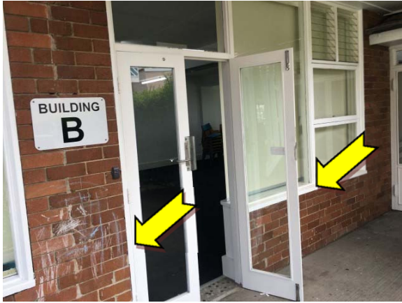
Photo 7. Exterior, throughout, window and door frames – suspected lead-containing white upper paint systems.
