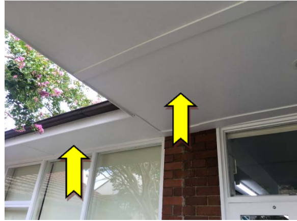
Photo 8. Exterior, throughout, awning and eaves – suspected lead-containing white upper paint systems.
