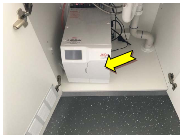
Photo 6. Interior, kitchen, below sinks, hot water boiler – suspected SMF internal insulation material.
