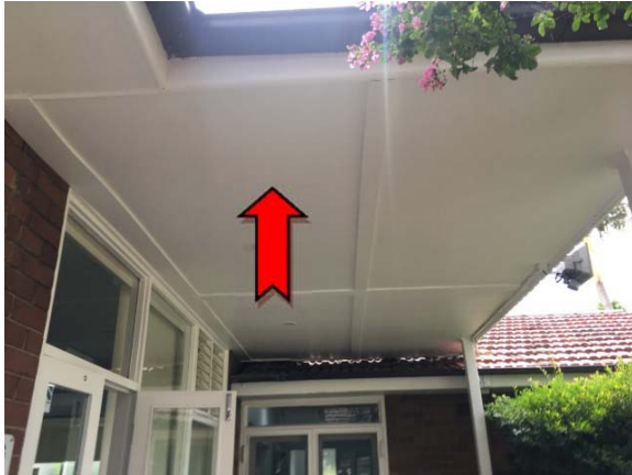
Photo 1. Exterior, throughout, awning – suspected asbestos-containing fibre cement sheeting.
