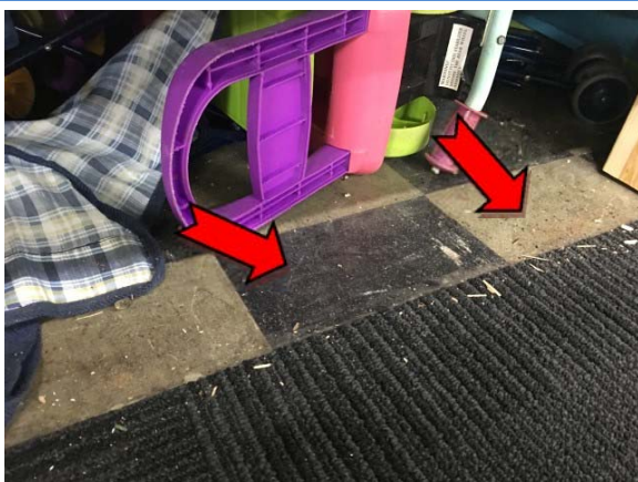
Photo 5. Interior, main hall, stage, subfloor, floor coverings black and grey – asbestos-containing vinyl floor tiles.
